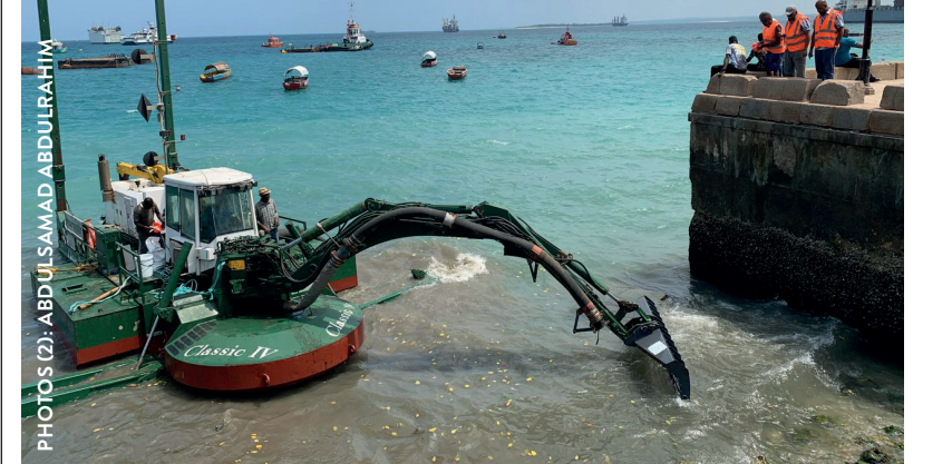
Heavy machinery removing stones from the sea; Abdulsamad Abdulrahim at the scene with officials and reporters (small photo above)
